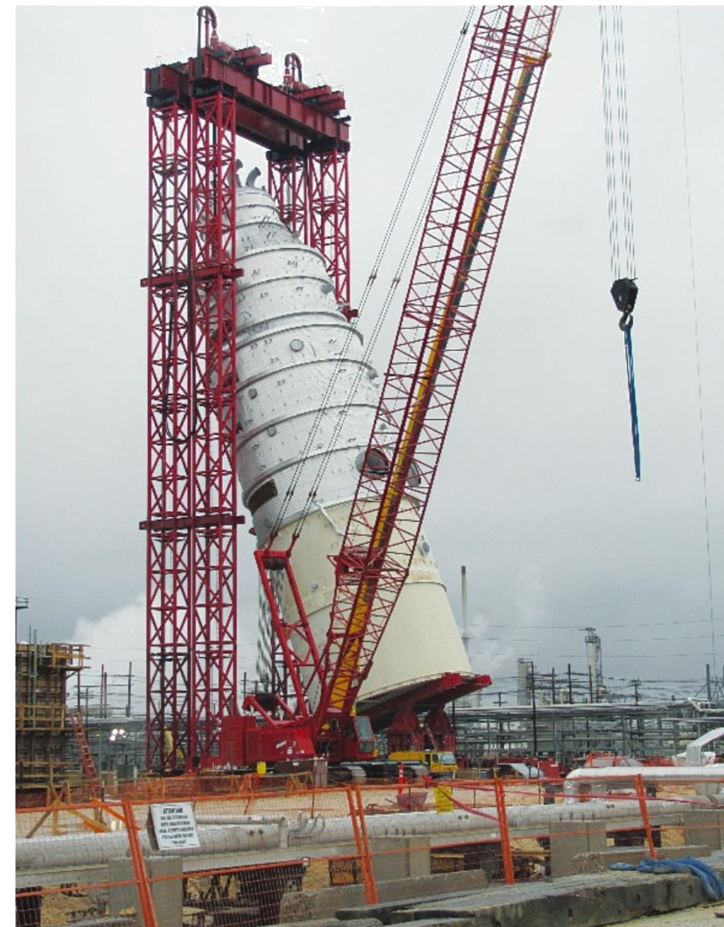
Crude Oil Processing Plant Expression
